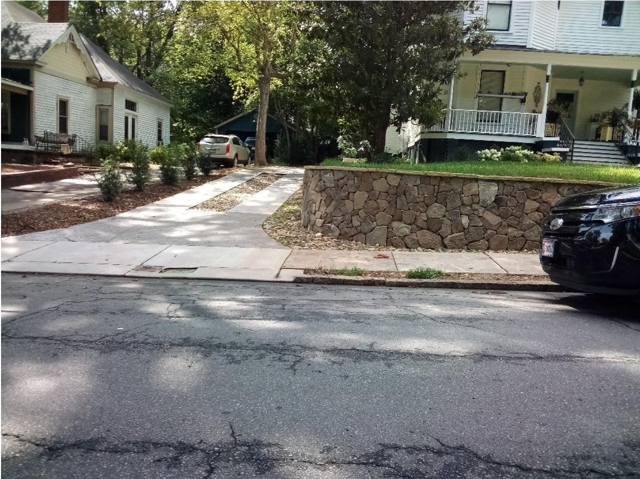
H-19-22 Existing Natural Stone Veneer & Cap - Tennessee Fieldstone Veneer on 74 Franklin Ave NW
